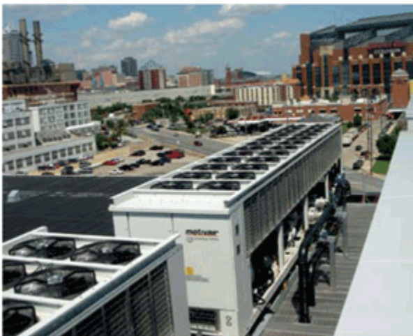
Air-cooled free-cooling chillers atop the LightBound facility.
