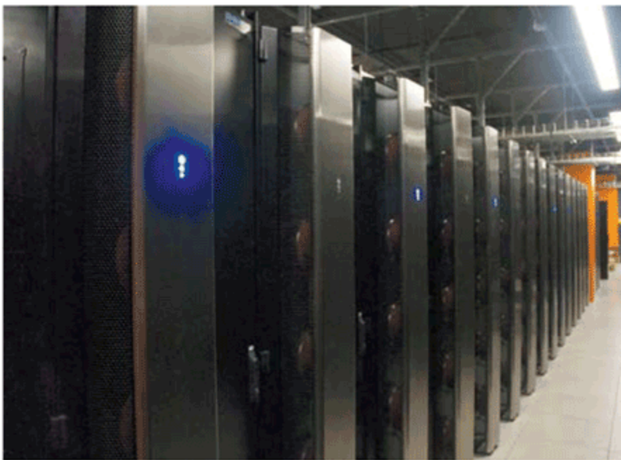
Chilled Door high-density rack-cooling units.
